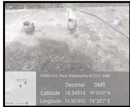
Rain Water Harvesting
